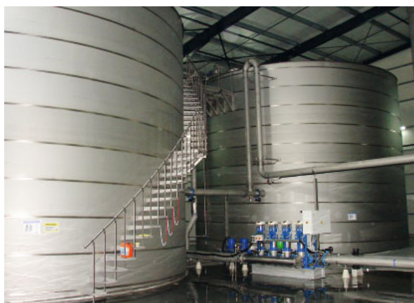
Fig. 3. Tank system with pressure booster system for pure water supply. © Hydro-Elektrik GmbH
